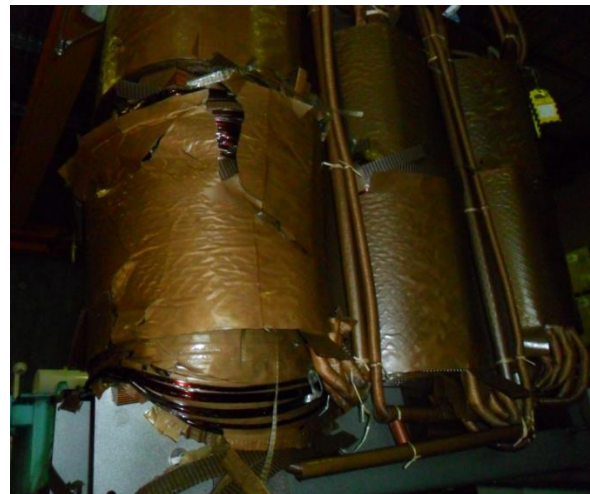
Fig. 4. Axial short circuit failure due to dynamic forces (mechanical failure).
